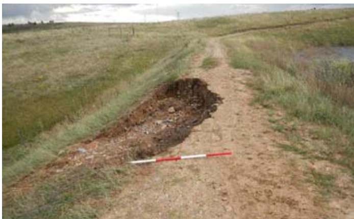
FIGURE 11 - PHOTO OF A SLOPE FAILURE CAUSED BY EMBANKMENT SATURATION DUE TO OVERTOPPING OF THE FLATIRONS VISTA DAM. THE WEAKENED DAM WAS EVENTUALLY BREACHED.
